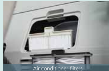
Air conditioner filters
