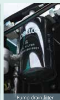
Pump drain filter
